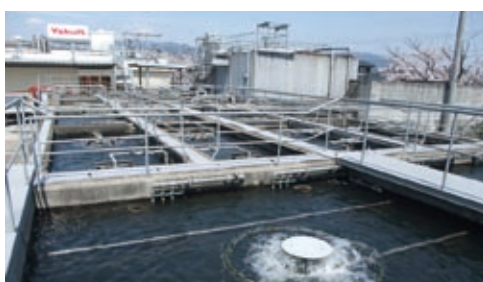
The Saga Plant's Yakult A&G Environmental Water Purification System in operation
