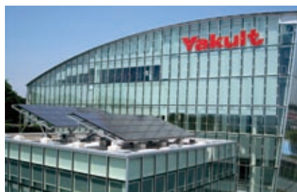
The expanded solar power generation system
