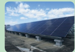
Solar power generation (Fukushima Plant)
