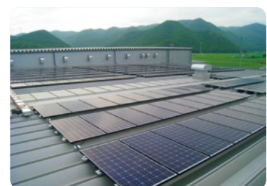
Solar panels (Yakult Okayama Wake Plant Co., Ltd.)
