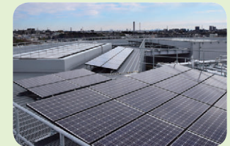
Solar panels at the Yakult Central Institute
