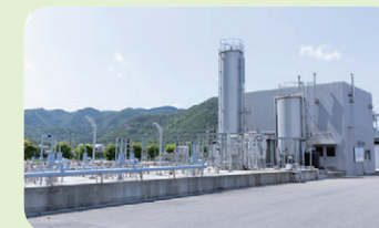
Wastewater treatment facility
