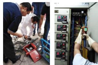
Electrical safety self-inspection at the Shanghai Plant
