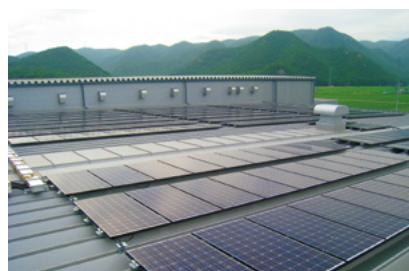
Solar panels (Yakult Okayama Wake Plant Co., Ltd.)
