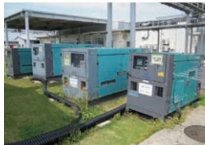
Generators at the Ibaraki Plant
