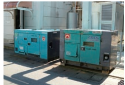
Generators at the Fuji Susono Plant
