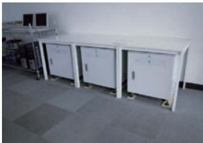
Lithium storage batteries at the Ibaraki Plant
